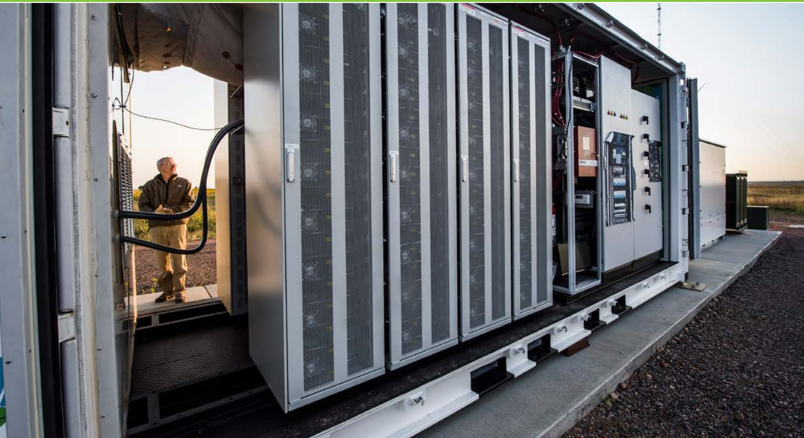
An employee opens the doors on the Flex manufactured battery enclosure, 1MW, 1 MWh rating, using lithium ion batteries from LG, at the Battery Energy Storage System, owned and operated by NREL for grid integration research at the National Wind Technology Center (NWTTC). Photo courtesy of U.S. Department of Energy.
