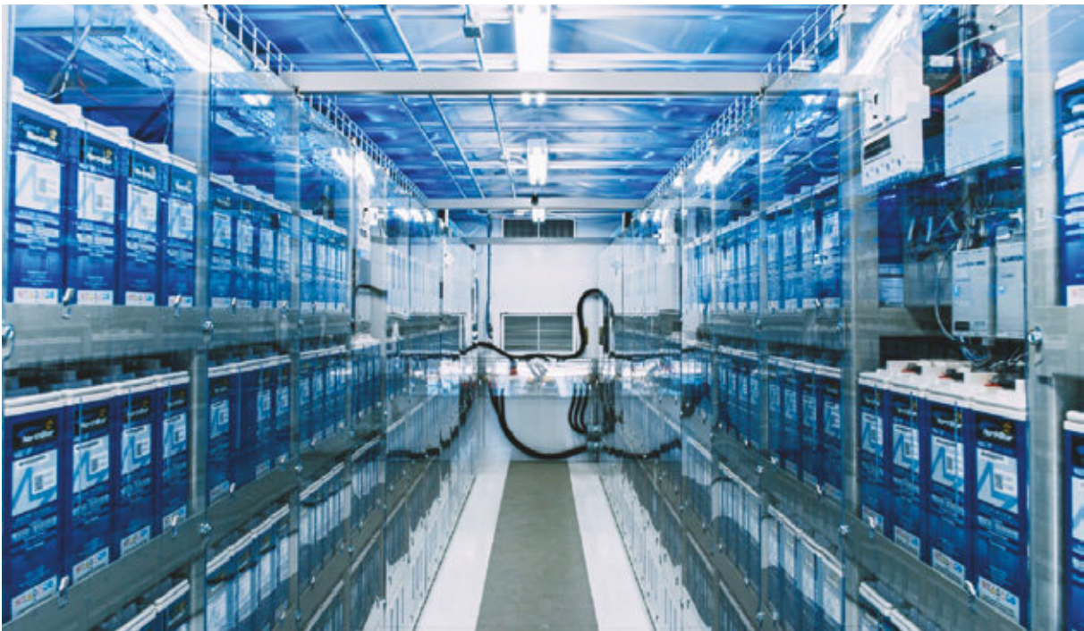
NorthStar Battery bank, Springfield energy storage project, Missouri, United States.
