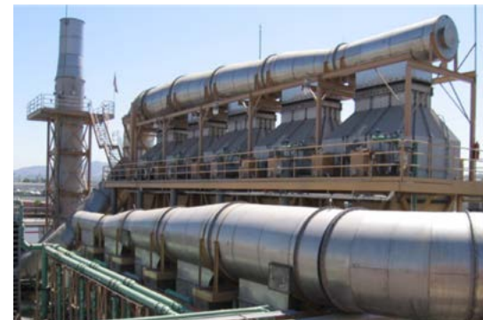
The environmental control system pictured cost the facility more than $25 million in 2008, creating significant benefits to the region by lowering emissions levels well below federal or state requirements.
